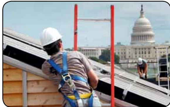
Stefano Paltera, US Dept. of Energy Solar Decathlon Iowa State student Timothy Lentz works on the roof of the Interlock House.
